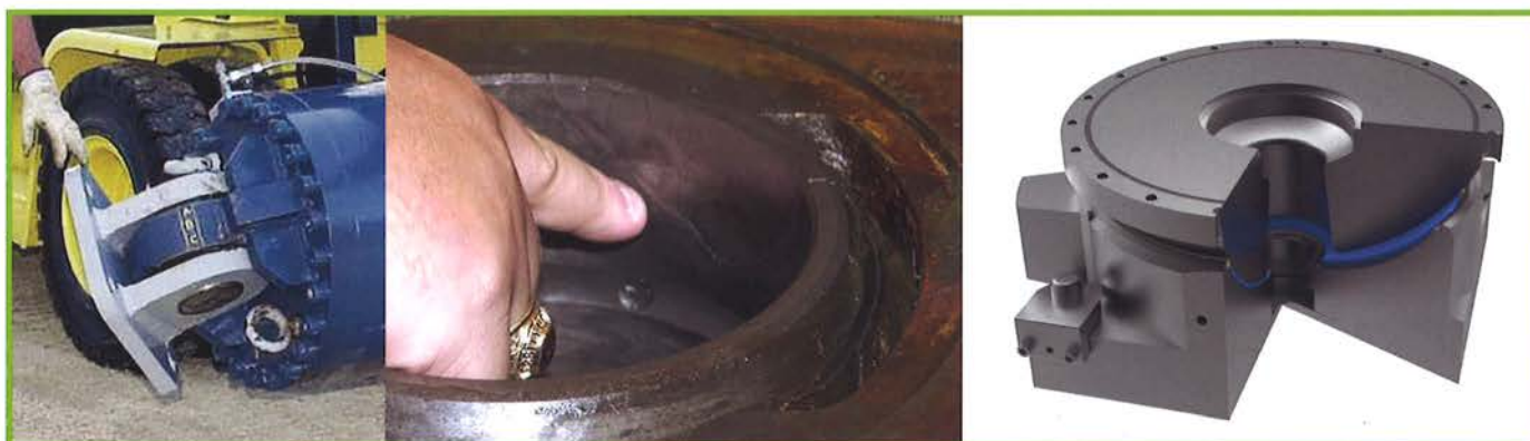
05 Old and cracked bearing and new bearing design with H- Glide lining
